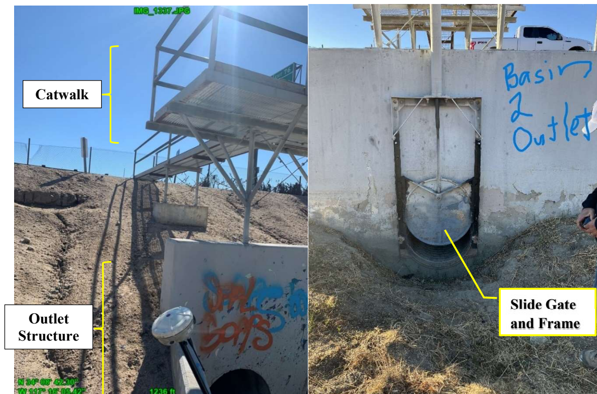
Figure 2.15 – Typical Existing Basin Outlet System with Outlet Structure and Catwalk
